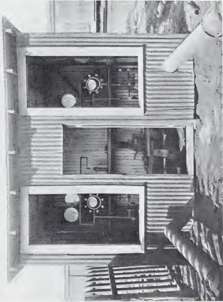
Fig. 6—ORIFICE METER INSTALLATION. "BOMBSHELL" TYPE GAUGES
